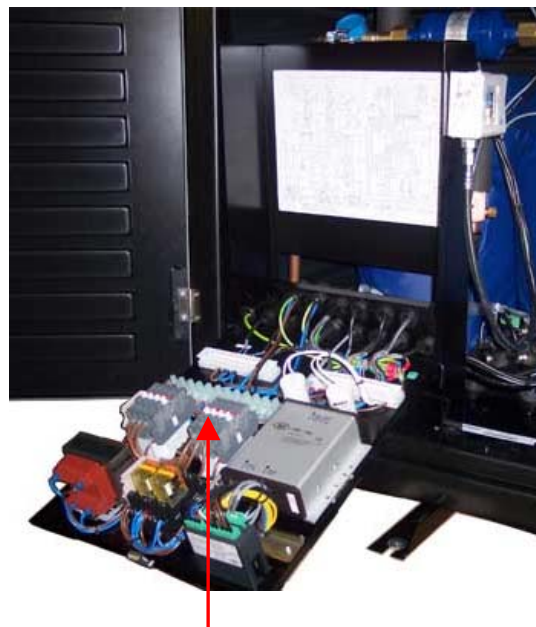
Contactor Access to the electrical components.
